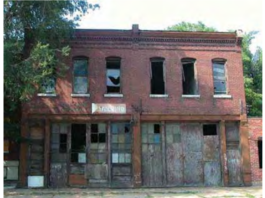
Lack of minimum maintenance over an extended period may render a building beyond rehabilitation.
