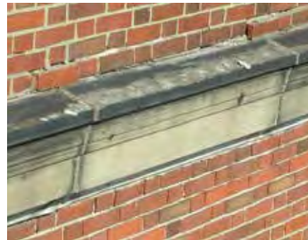
Loose brick due to poor conditions of mortar joints (moisture and movement in masonry system).
