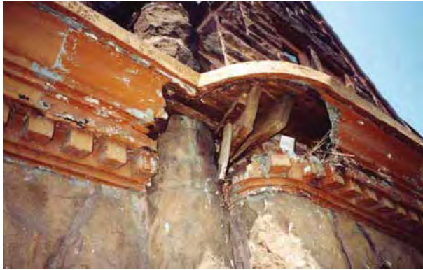
A painted lead-coated copper cornice is missing elements due to advanced deterioration of metal.
