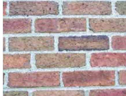
Damage to brick caused by sandblasting.
