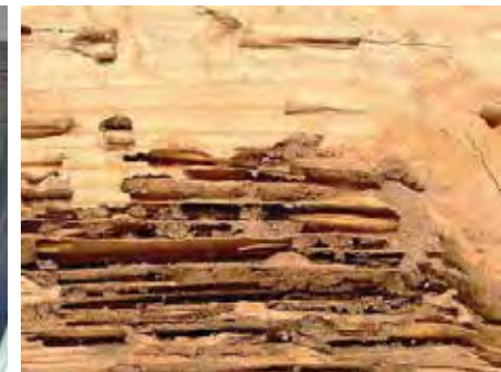
Galleries and debris in a wood floor joist indicate insect infestation.
