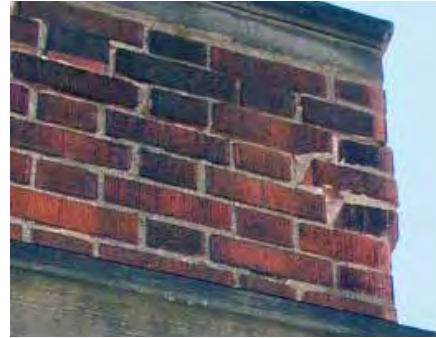
Displacement of brick by movement in the parapet wall.
