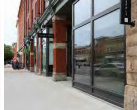
Far left and middle: Sidewalks were graded, and a sloped sidewalk was installed to create a gentle ramp that makes the building accessible without negatively impacting the appearance. Right: Accessibility was created from the street corner to the building entrance by sloping the sidewalk to have a zero profile edge at door entry and curb.
