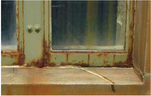
Corrosion/rust on a steel window sash resulting from exposure to moisture and air.
