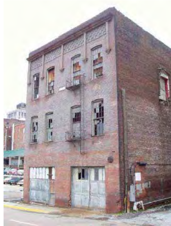
This structure has been neglected and is not dry or safe.
