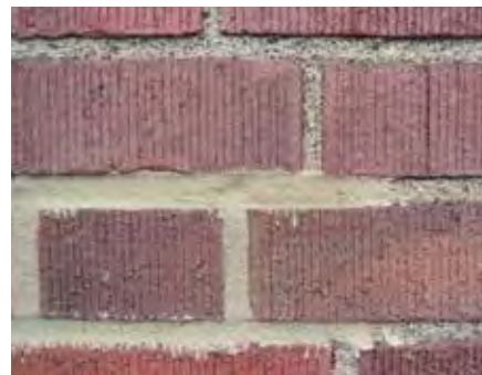
Recent poor repointing. New mortar has been smeared onto the face of the brick and does not match original mortar in color, texture or tooling.
