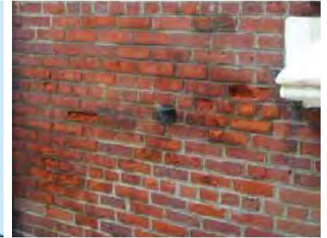
Deterioration of brick caused by moisture is marked by discoloration and brick erosion.
