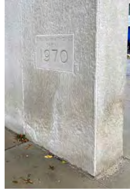
Foundations may exhibit efflorescence as a result of damage from salt-based snow removal chemicals.
