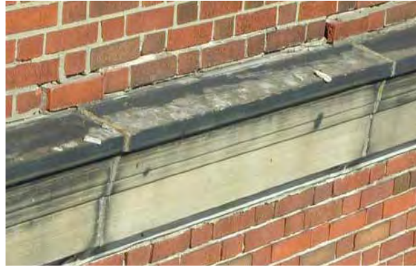
A loose stone cornice attached by metal fasteners indicates that its fasteners have failed.
